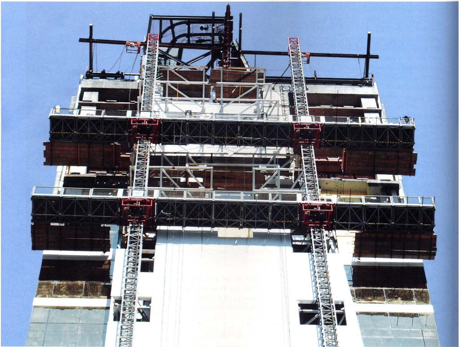
Northeast Mast Climbers provided access to an area that was over 470 ft high and 60 ft wide.
