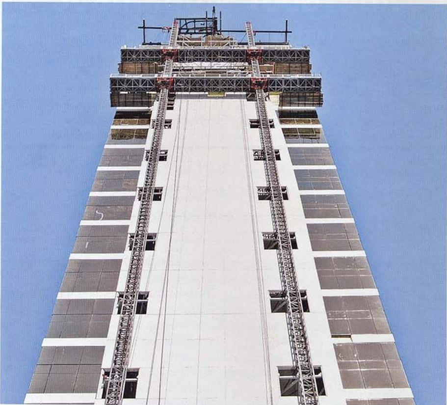
A fire at the Borgata Hotel & Casino destroyed the south façade of curtain wall and panels.
